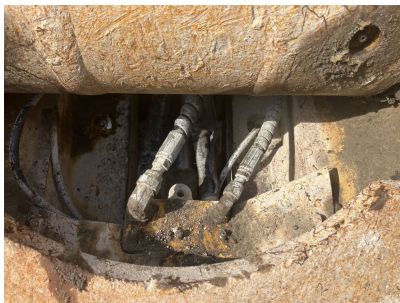
Image Comment(s): Coupler cover missing. Grease lines damaged.
