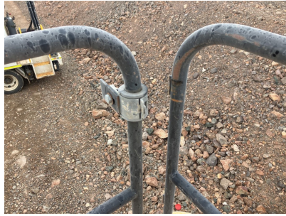
Image Comment(s): Handrail damage.
