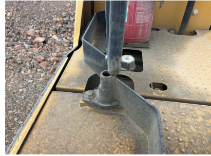
Image Comment(s): Handrail damage.
