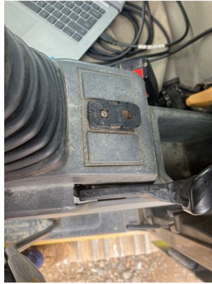
Image Comment(s): Switch cover missing.
