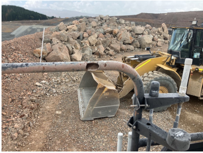
Image Comment(s): Handrail damage.
